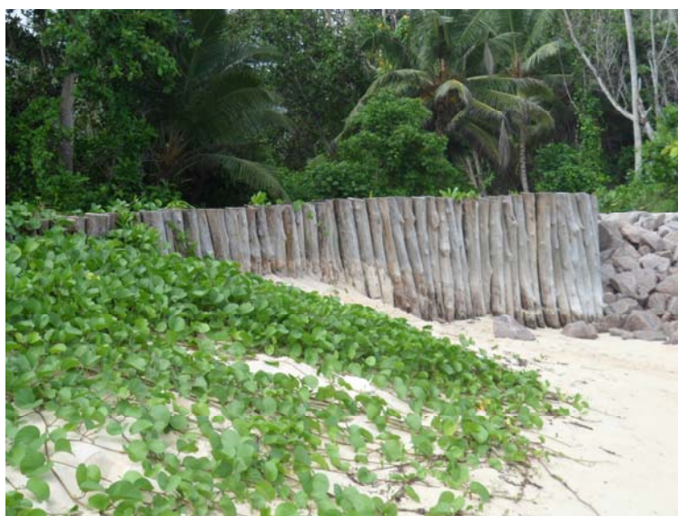
Photo [Stavros Mavrogenis]: a sea wall made of causarina trees pillars in Mahe island, Seychelles
