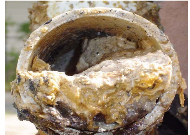
Consequence of dropping oil in sewer
