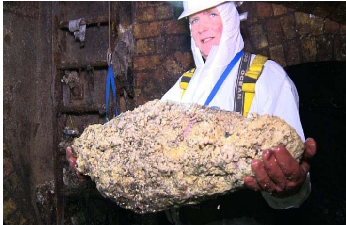
Sewer blockage in UK costing €20m
