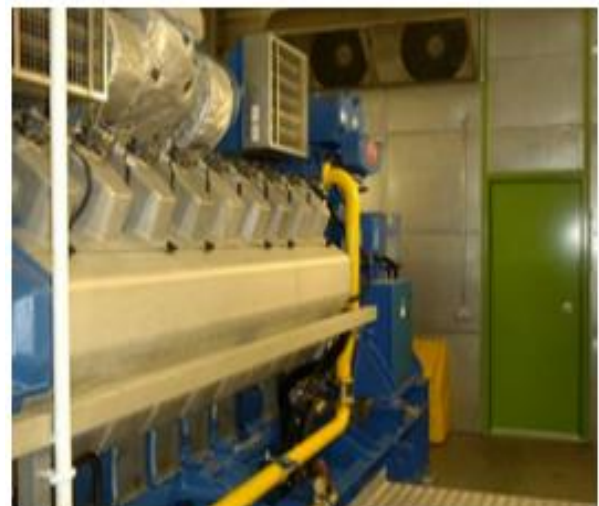
Figure 4 Internal combustion engine CHP plant Source- Carbon Trust
