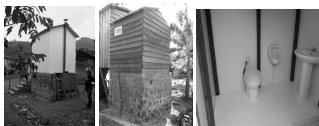
Figure 2. ECOSAN bathrooms installed in Neves
