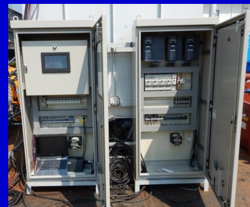
Photo of Control panel
